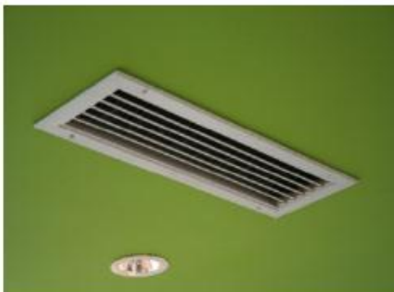
Diffuser air vents
